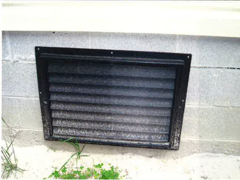
Type of Engineered Vent 05/06/2013
